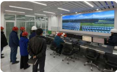
Prefabricated Secondary Equipment
