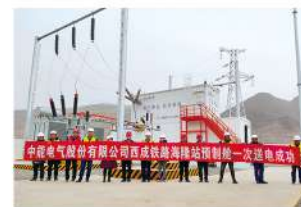
110kV Xicheng Railway Prefabricated Substation
