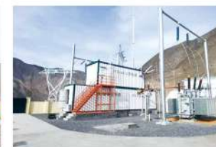
110kV Xiahe Prefabricated Substation
