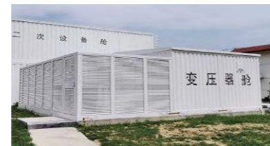
Secondary (Control, Protection) Cabin & Transformer Container
